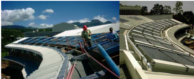
Solar Cooling 35 kW 2003
